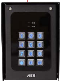
Gate/Entrance 4 Auxiliary Prox & Keypad Unit
