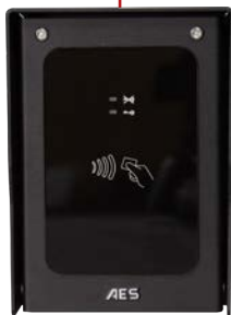
Gate/Entrance 3 Auxiliary Prox Unit
